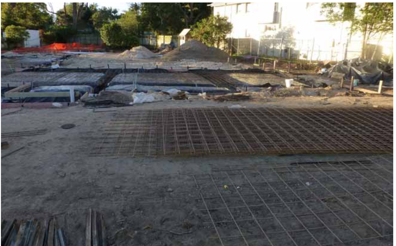
BELOW: Steel reinforcing for concrete slab stacked up and worked on outside the footprint of the concrete slab being constructed. Construction zones for building concrete slabs can be 2 to 5 metres wide but are often much wider even on relatively flat ground as at this site in The Parapet, Castlecrag which until recently had a beautiful garden.
